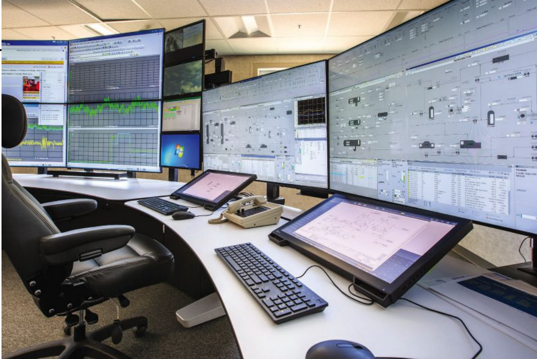
Figure 2: A modern control system is an opportunity to bring people, the plant and data together to drive better business. Honeywell Experion Orion Console is the most advanced and cyber secured control system, according to Honeywell Process Solutions.
